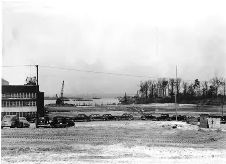
Naval Air Station, Patuxent River, MD. Seaplane Hangar (Steel), Trans. Area. (Project No. 4). View Looking north showing apron. Contractor Cummins Constr. Corp. and Riggs-Distler and Co. Contract NOy-5363. Date 3-1-1943 (PW# 1199)
