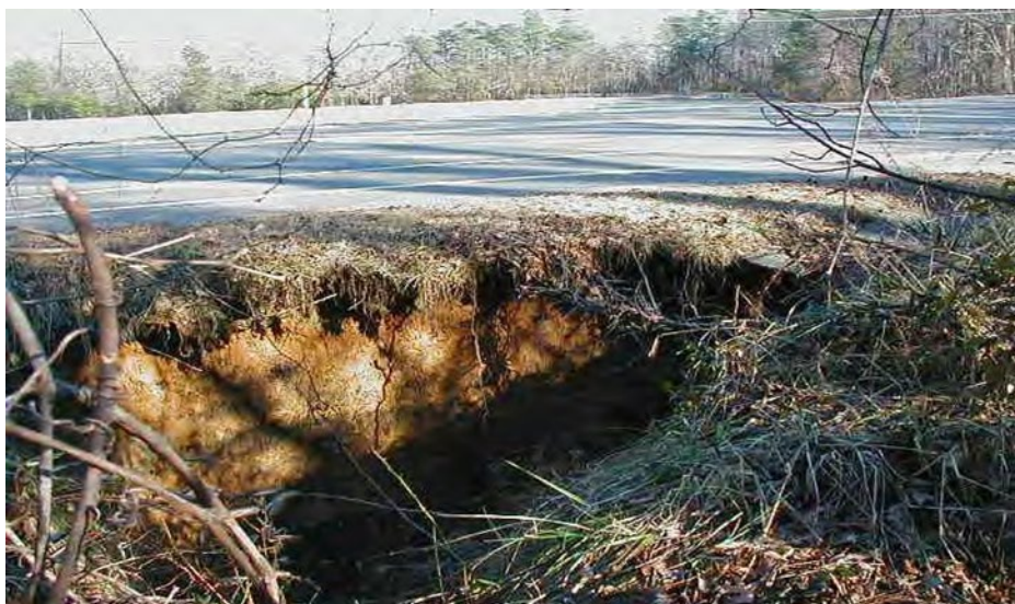
Example of erosion at PAX; Stormwater management will help remedy similar future impacts.
